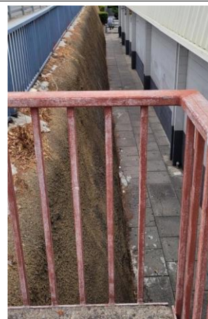
Figure 5: [Vicinity Centre] slab path may have minor lips and gaps
